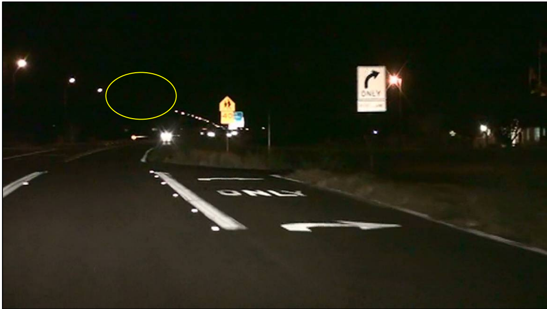
Gap in lighting created by malfunctioning street lights near the rest area
